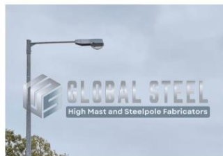
Street Light Steel Poles
